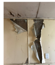
Water damage to an internal wall
