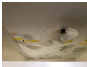
Mould growth to toilet ceiling
